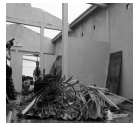
Damage due to typhoon 12
